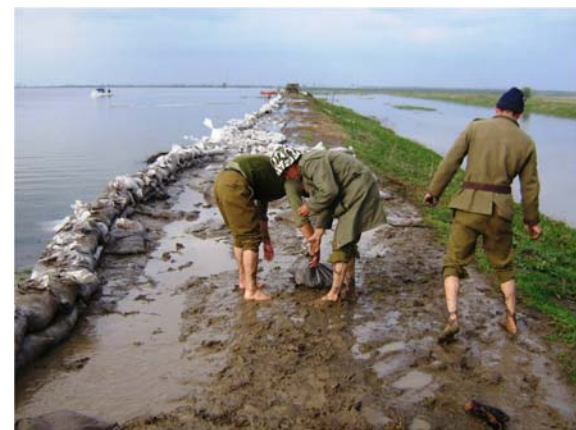
Dyke protection work (source: Romanian Waters)
