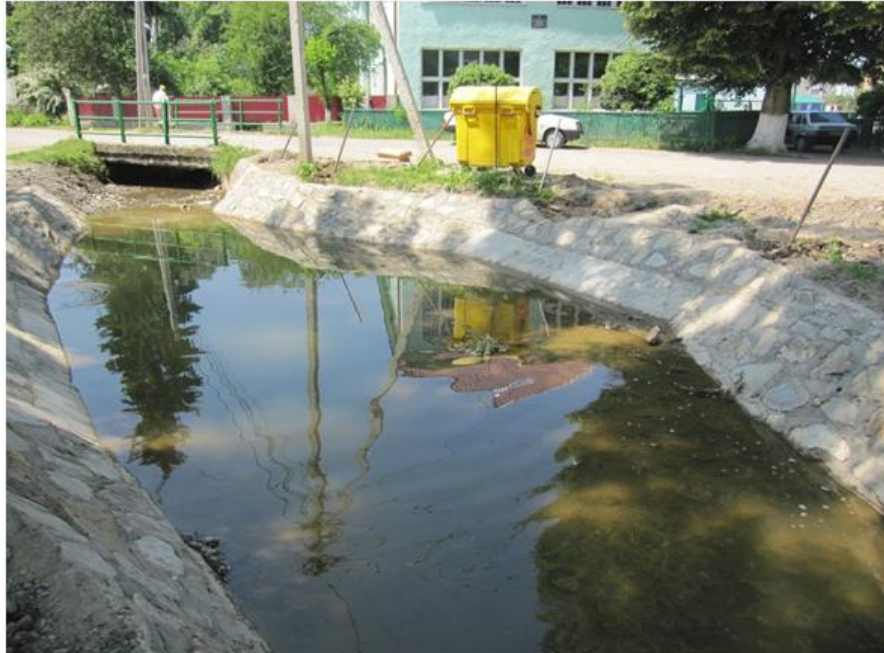
Sediment catcher before the first bridge in lowland part of the village
